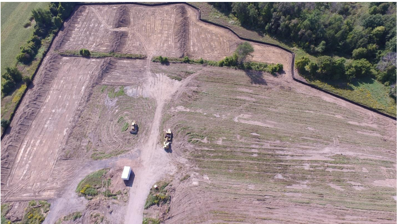
Viewing West, established silt/sediment control fencing, clearing, grubbing and removal of fill
