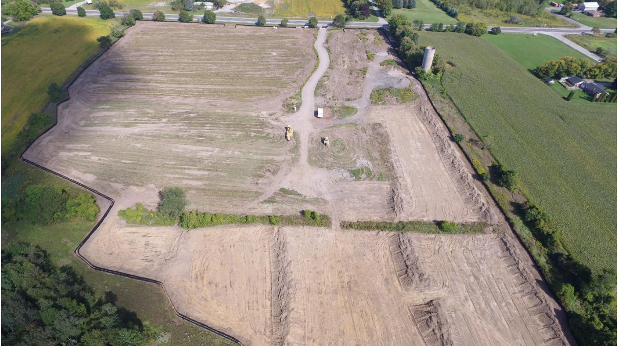
Viewing East, established silt/sediment control fencing, clearing, grubbing and removal of fill
