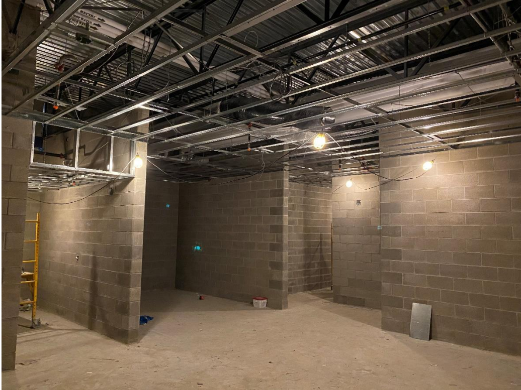
Electrical distribution and “t” bar ceiling in Men’s changeroom
