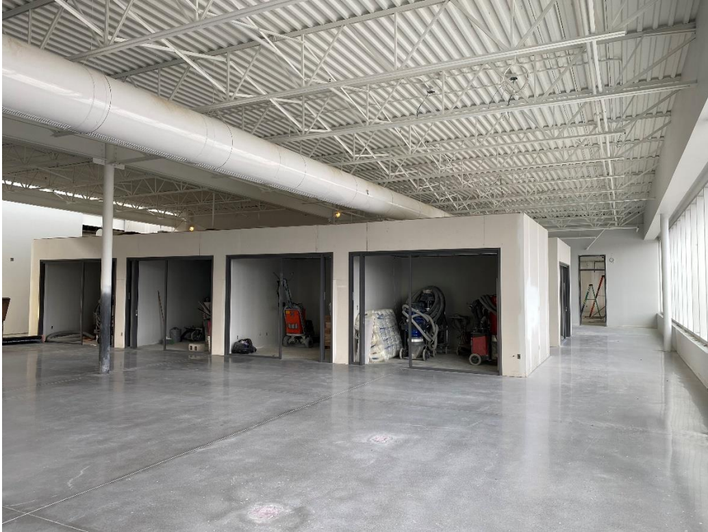
Painted ceilings and polished flooring of private offices in the administration area
