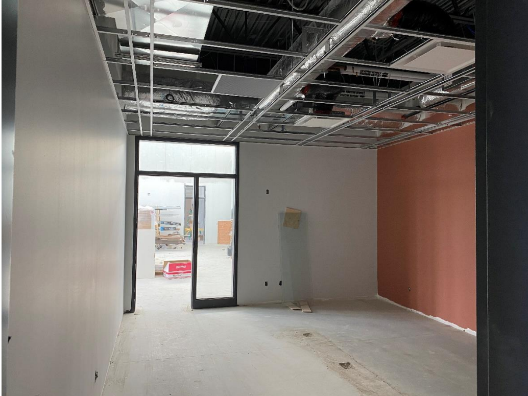
Accent painting and "t" bar ceiling in the administration area meeting room
