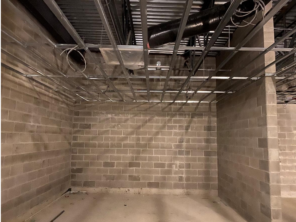
Electrical distribution and "t" bar ceiling in Women's changeroom
