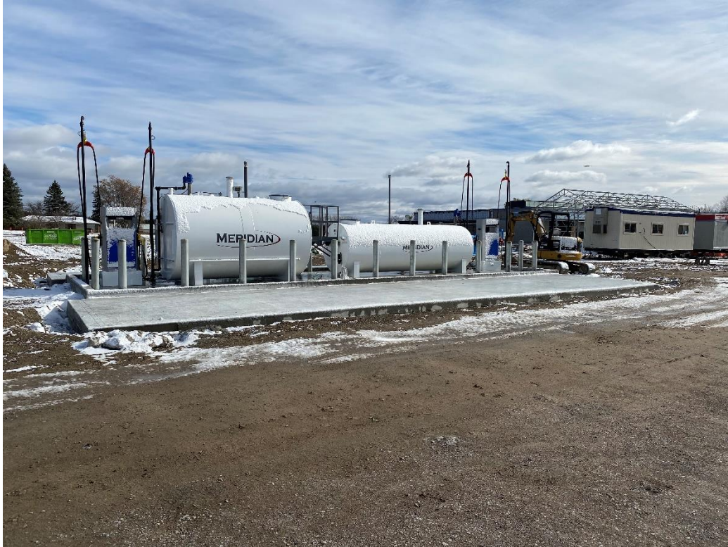
Installation of fueling island, tanks and pumps north end of the site
